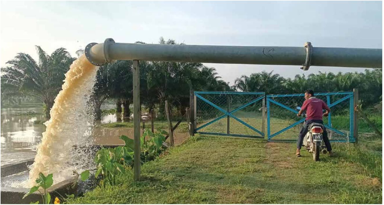
The Bukit Tadam JPS officer (and villager) carrying out his daily rounds - monitoring Sungai Langat levels and existing village mitigation efforts including this pump. Photo from Bukit Tadam Facebook page
